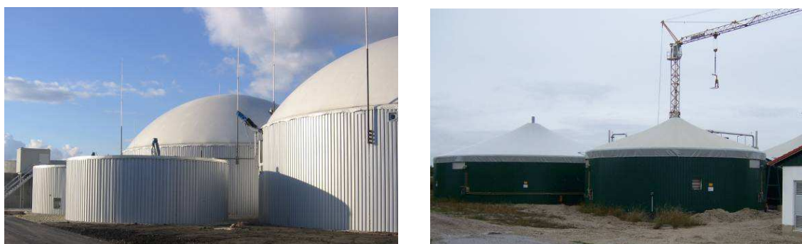
Figure 7.20 Vertical digesters, covered by gas proof membrane. The membrane top is inflated by the produced biogas –left (AGRINZ 2008); The membrane top is fastened to a central mast –right (RUTZ 2006)
