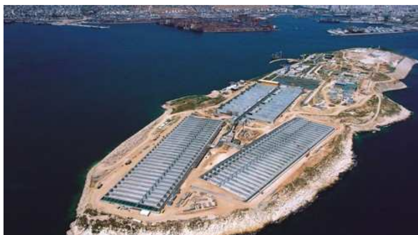
Figure 4.11 Waste water treatment plant in Psyttalia, Greece (FARNSWORTH 2004)
