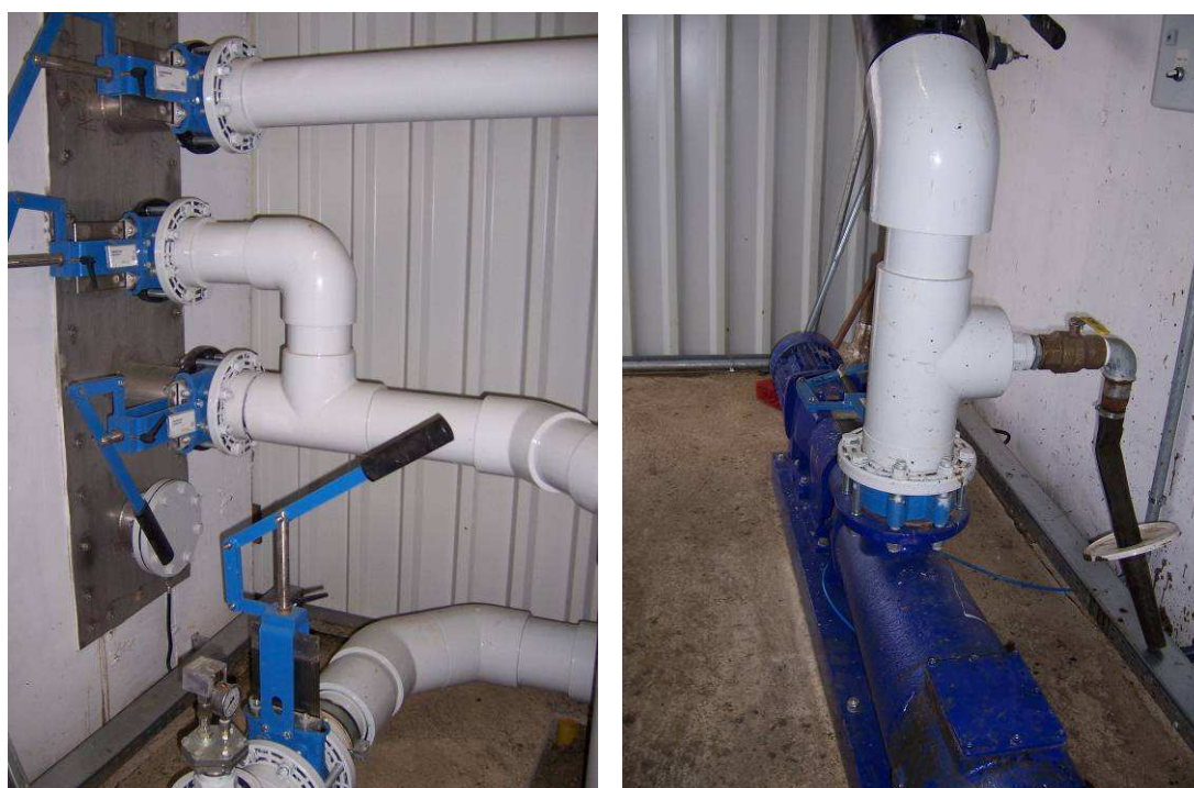
Figure 7.8 Stop-valves ( left ) and pumping system ( right ) (RUTZ 2006)
